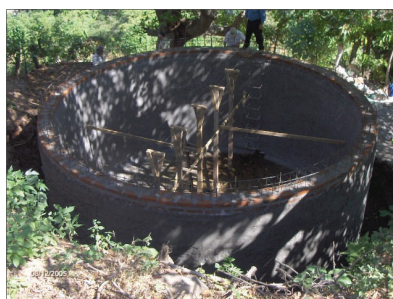
water tank in san jose el naranjo
